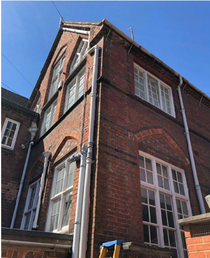
East Facing Gable, line of former flue just visible on north facing return brickwork
